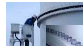
ENERGY (WIND POWER)
